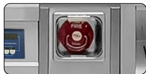
Ansul Fire Suppression System
